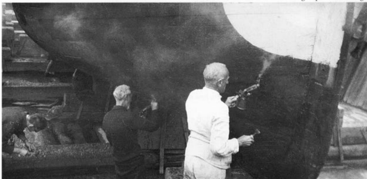
Volunteers working on the Plane scraping off the hull at Fellowes yard, Yarmouth
